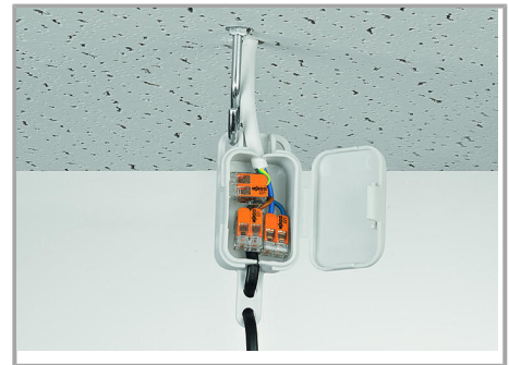
Pendant light connection in suspended ceilings
