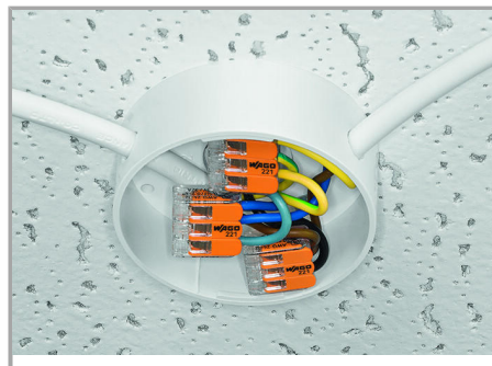
Lighting distribution in ceiling canopy
