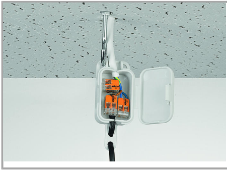
Pendant light connection in suspended ceilings
