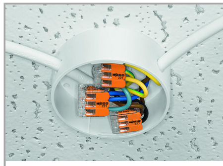
Lighting distribution in ceiling canopy
